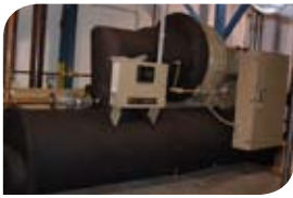
A Trane CenTraVac™ chiller installed at Ocean Spray facilities.
