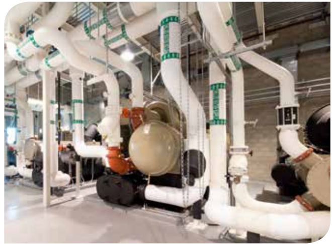
A 900-ton ultra-high-efficiency Trane® CenTraVac™ centrifugal chiller was installed to increase capacity of the LAC chiller plant.
