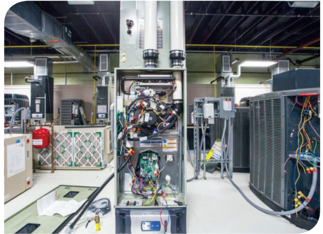
The Hill College lab consists of everything students need to be well trained in various aspects of commercial and residential HVAC.
