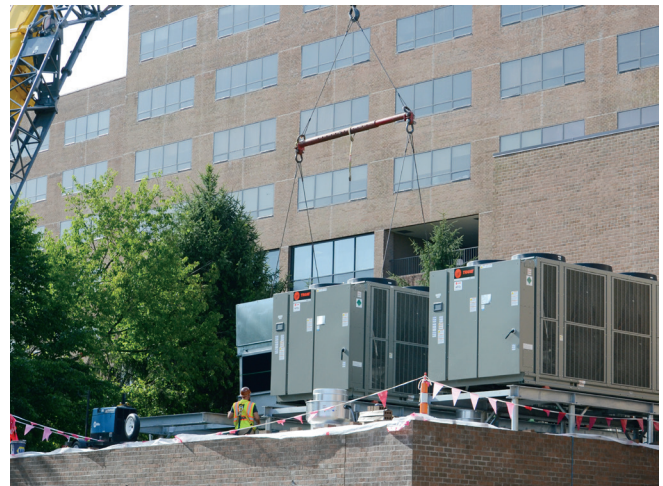
Two Trane Stealth air-cooled chillers provide efficient, quiet operation to generate ice at night for the Norton Audubon thermal storage system, shifting demand load to lower-cost, off-peak hours.
