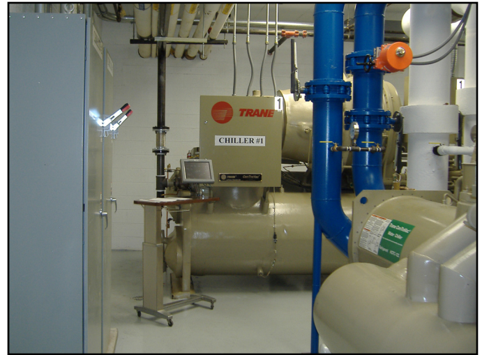
Two high-efficiency Trane CenTraVac® centrifugal chillers replaced aging equipment in the hospital's chiller plant to reduce energy use.
