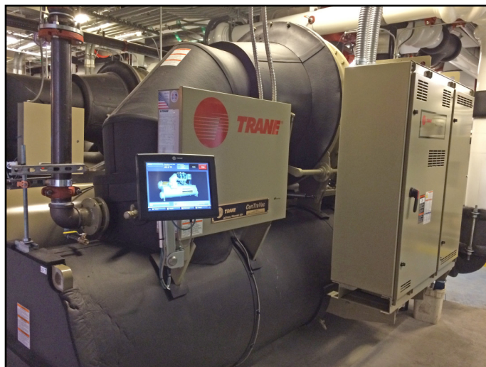
Asante Rogue Medical Center added a 500-ton Trane® CenTraVac™ chiller with Adaptive Frequency™ drive to improve redundancy and efficiency.
