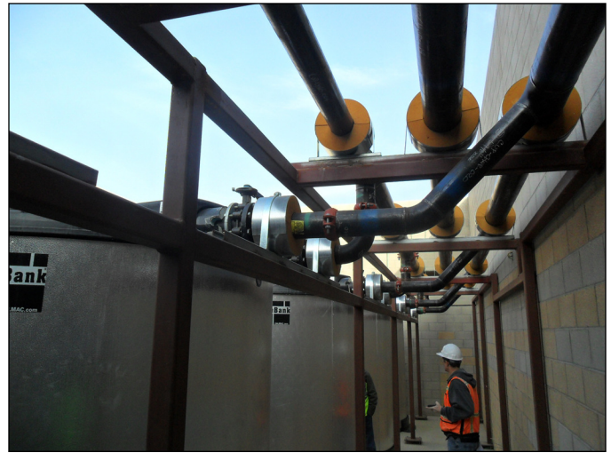
CALMAC thermal energy storage shifts load to less expensive nighttime rates to help reduce energy costs.
