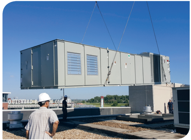
Two 70-ton IntelliPak rooftop units provide efficiency and comfort for the brewery's tour and tasting facility.
