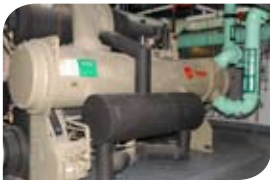
One of three 800-ton Trane chillers installed at 11 Madison Avenue as part of a thermal storage system.
