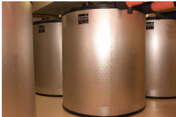
48 CALMAC ice storage tanks
