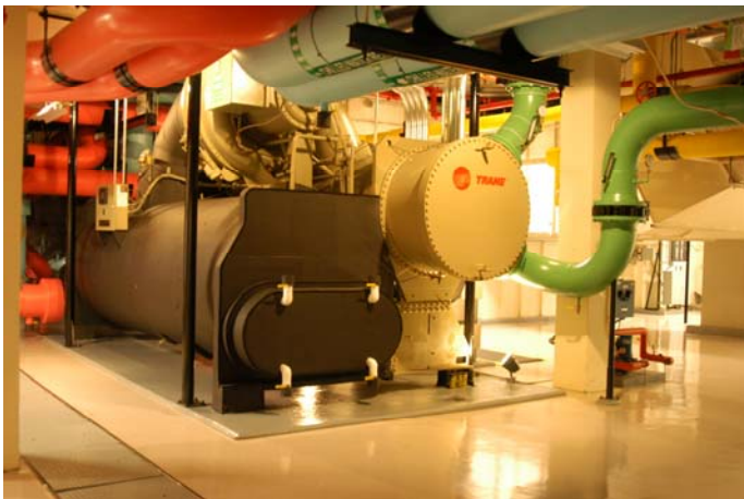
Trane 1400 ton CentraVac centrifugal chiller is part of a thermal storage system
