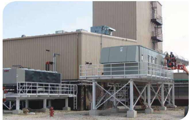
The Solae Remington plant includes a five-story packaging tower.
