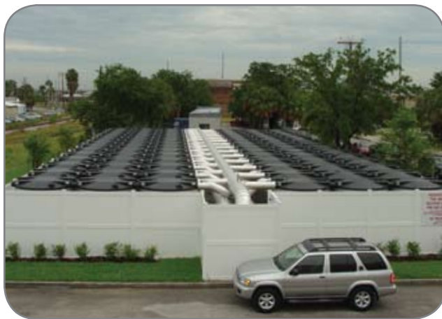
Hillsborough County Facilities
