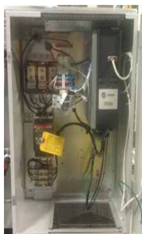
Figure 126. Externally mounted VFD
