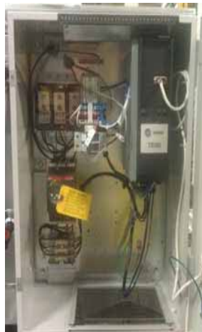
Figure 122. Externally mounted VFD
