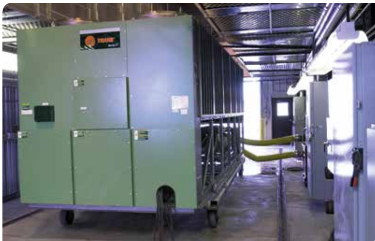
On-site test facility ensures reliability and performance verification
