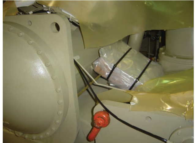
Figure 30. Power cable and Ethernet cable connections
