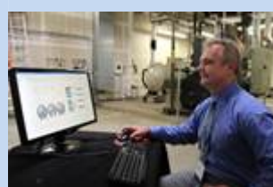
Gene Archer, technical services manager for FSSI, demonstrates the Trane Tracer Summit™ Building Automation System (BAS).
