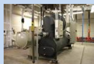
The 168,000 square-foot FSSI headquarters uses two Trane chillers to handle cooling, including a 400-ton Trane centrifugal water-cooled chiller and a 100-ton Trane Series R™
