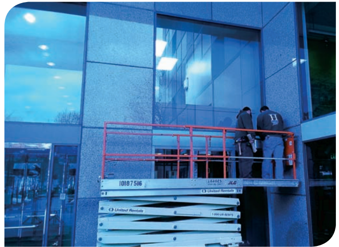
The on-site R'newal service team worked diligently in the early morning hours, removing a large window to accommodate component replacement.
