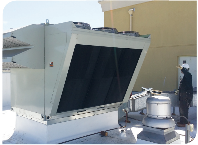
The Trane® Horizon™ dedicated outdoor air systems installed on the roof filter 100 percent outdoor air to improve indoor air quality.
