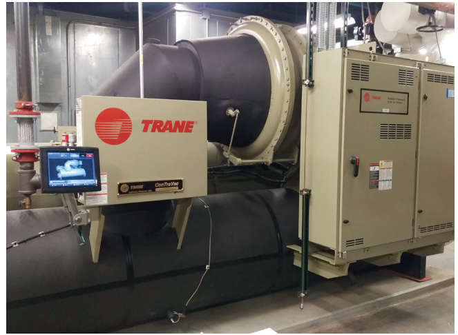
Trane technicians spent eighteen months fixing, repairing and replacing more than 3,200 pieces of equipment at thirty-two District schools.
