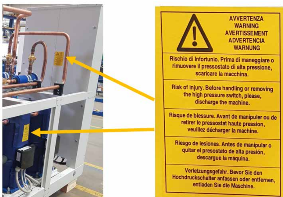
Figure 2- Indicative position of the signs warning about the necessity of replacing the high pressure switches with the unit void of refrigerant
