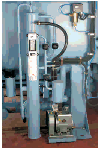
The Purge System
