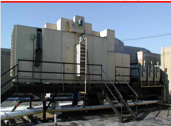
EXISTING WAHLSTROM MAKE-UP AIR HANDLERS BEFORE RENOVATIONS
