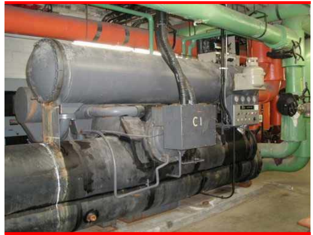
EXISTING WAHLSTROM CHILLERS WITH NEW DDC PANEL
