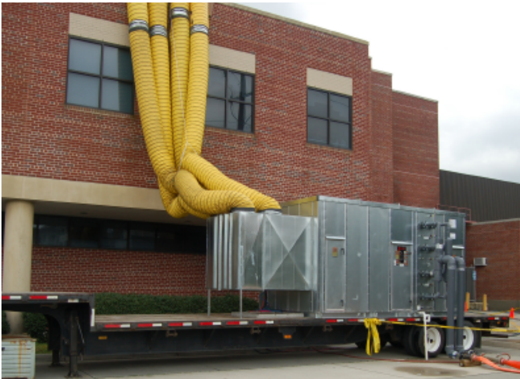
Temporary air handlers being utilized.
