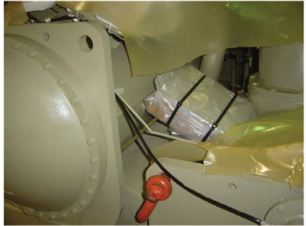
Figure 30. Power cable and Ethernet cable connections
