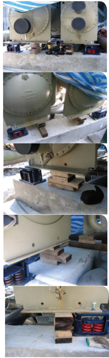
Remember! this is an example of what NOT to do. INCORRECT Spring Isolator Installation.
