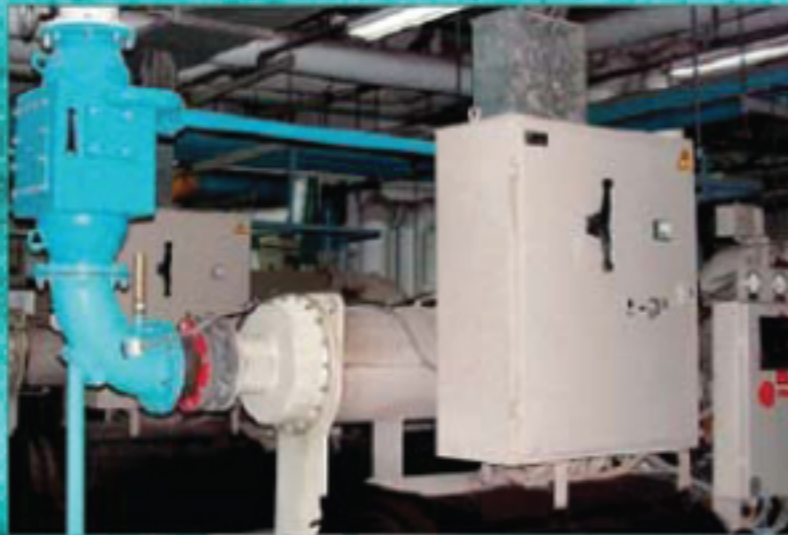
▽ Tube cleaning system installed on Trane CVGD chiller
