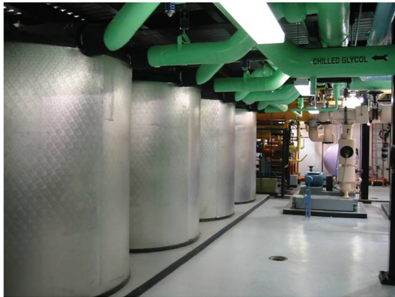
FIGURE 3 Thermal energy storage tank capacity.
